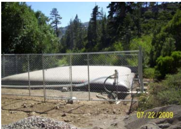
Bladder used for water storage at tank construction site
